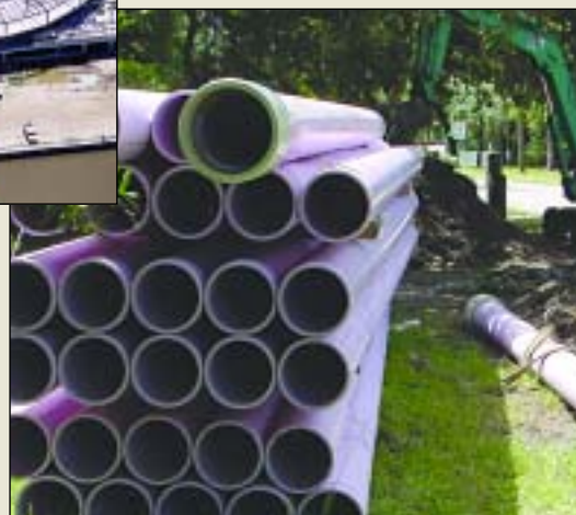
Miles of pipe are being laid to provide reclaimed water service to Clearwater residents.
