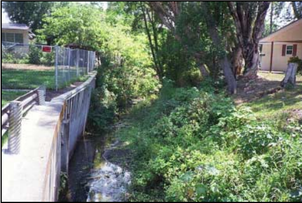
Figure 3.1-20. Failing Retaining Wall Upstream of Browning Street, to be Replaced and Exotic Vegetation to be Removed
